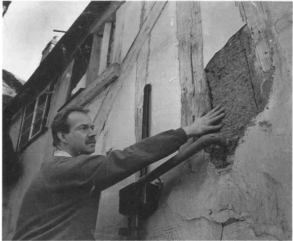
Doing a repair the traditional way - Christopher North testing a re-daubed opening before applying the first coat of lime render.
